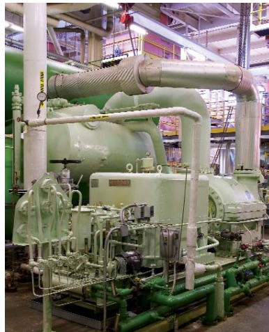
Murray Turbines Drive Chillers at UWM's Power Plant
