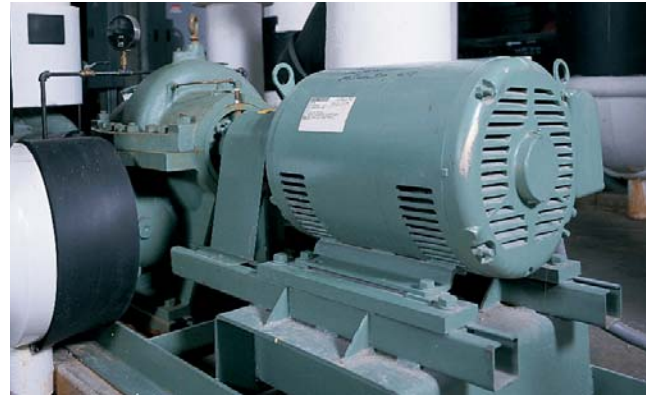
This Motor Drives a Taco Horizontal Split Case Pump at the Midwest Express Center
